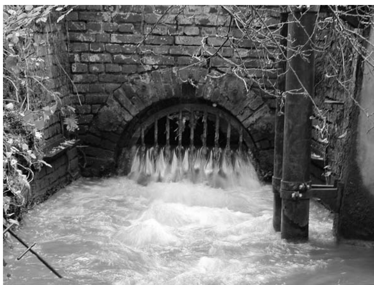
Fig. 11: The portal of the 7.5 km long German Burgfey/Eifel mine water adit discharging 15—19 m 3 min -1 of polluted mine water of the abandoned Mechernich mining area into the Veybach stream.
