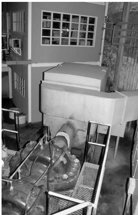
Fig. 28: Mine dewatering pump and mine water scheme control room in the Vazante/Brazil underground zinc-mine.
