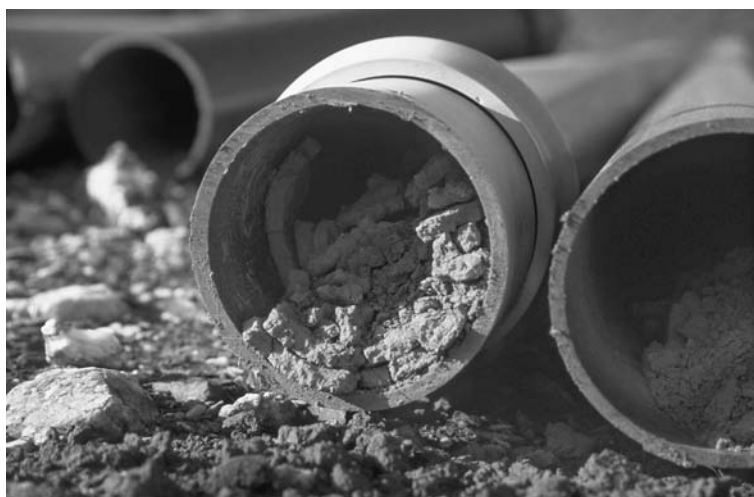
Fig. 7: Ochre precipitates in a mine water discharge pipe of the abandoned Straßberg/Harz fluorspar mine.
