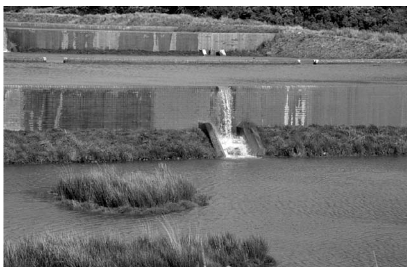
Fig. 91: Mine water overflowing the Pelenna II/Wales system. The hydraulic head is too low to drive the water through the compost (March 24 th 2000).
