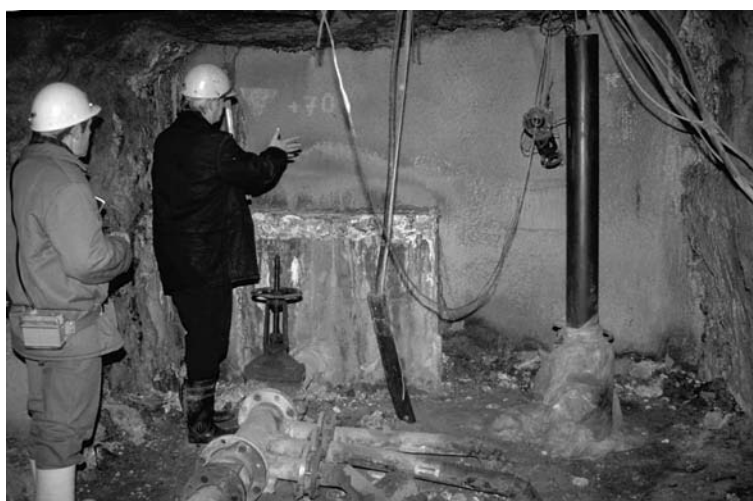
Fig. 22: An underground dam in the abandoned Königstein/Germany ISL uranium mine to prevent the discharge of highly acidic leachate fluid (January 8 th 1992).
