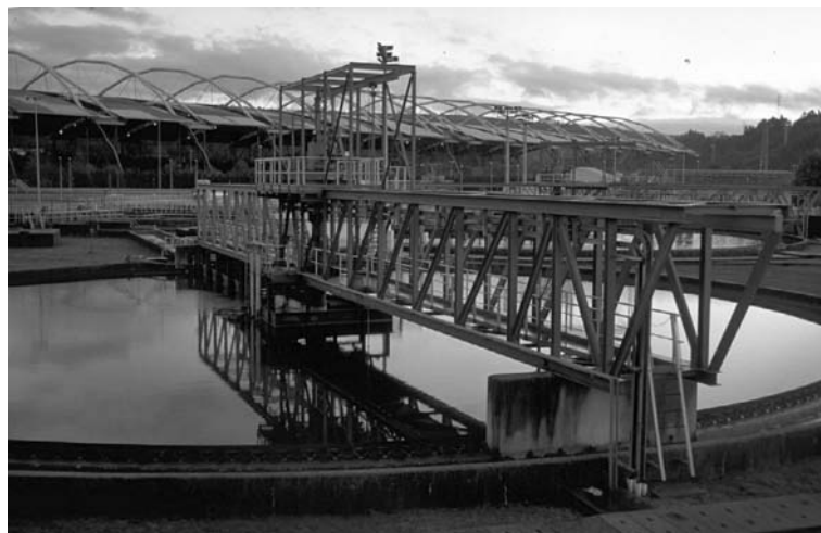
Fig. 88: Radial flow clarifier of an active mine water treatment plant at As Pontes lignite mine (Spain).
