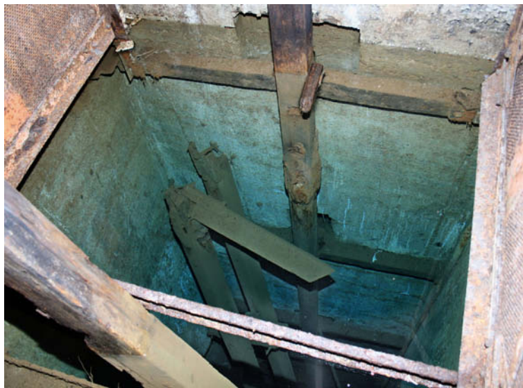
Fig. 36: Rotten shaft furniture in a flooded shaft of the closed Schwaz/Austria dolostone mine. The water surface is just a little bit below the left corner of the shaft.
