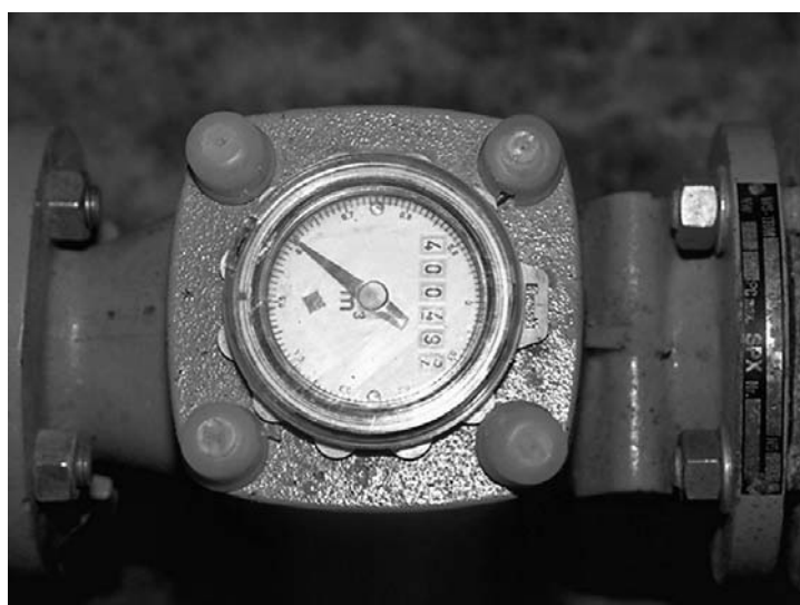
Fig. 59: Mechanical, propeller based water meter at the abandoned Dienststelle Marienthal bunker near Marienthal/Germany.
